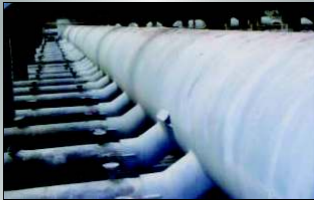
Zuyevska Thermal Power Plant – Ukraine
