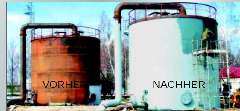
Kobrin Oil Pumping Station – Belarus
